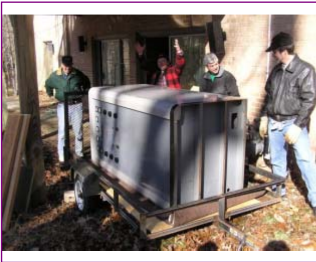
PHOTO 2: The BC-250GY transmitter removed from KOBRA's shack and loaded onto a small trailer, ready for transport up a grassy slope using manpower and a block & tackle secured to a suitable tree.
